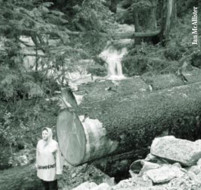
Interfor road construction in Johnston River (spring 1998) to provide logging access into the intact Johnston Creek watershed.
