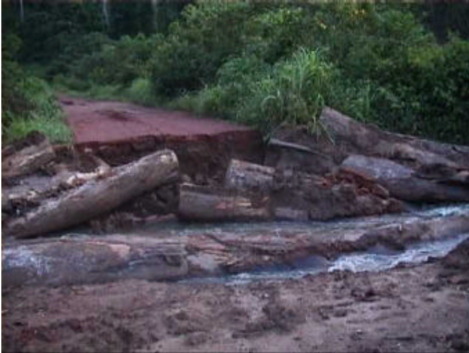
Photo: Broken bridge: preventing access to SFH-concession UFA 08-003 / © Global Witness / june 2000
